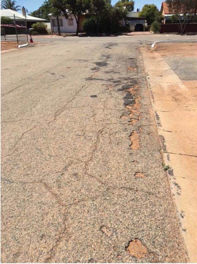
Above: Memorial Ave requiring patching and sealing
